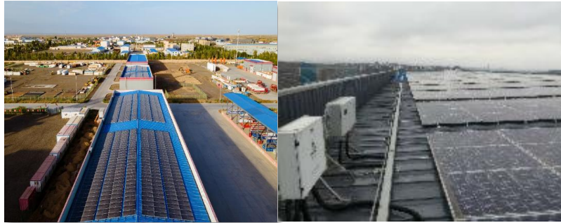
▲ Tarim Drilling PV Power Generation
