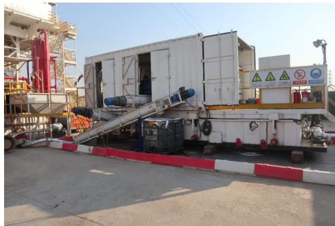
▲ In situ reduction device of oil-based drilling cuttings
