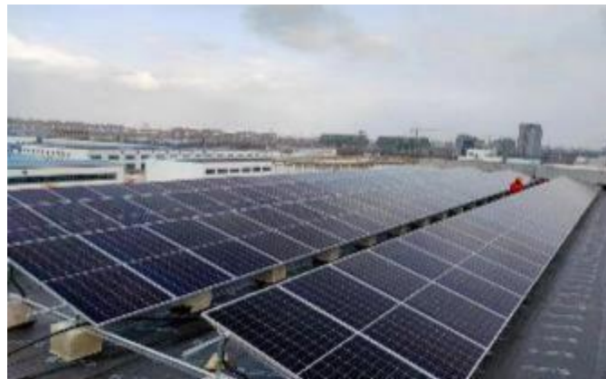
▲ PV Power Generation at the Pipe Technology Service Center
